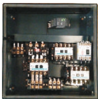
Interior View of MU-G20W FASD
