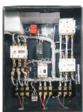
Interior View of MU-G30W FASD
