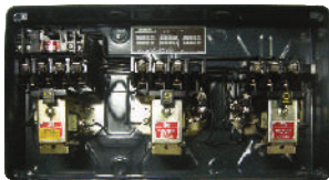
Interior View of MK1 SASD
